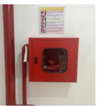
Fire Hose Reel
