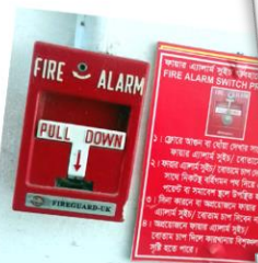
Fire Alarm Switch
