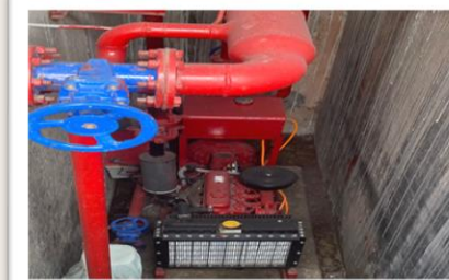
Hydrant Pump Room
