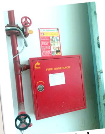
Fire Hose Rack
